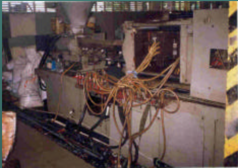
Oil Leaks & poor House Keeping Practices
