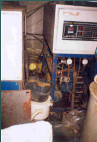
Oil Leaks & Poor Maintenance
